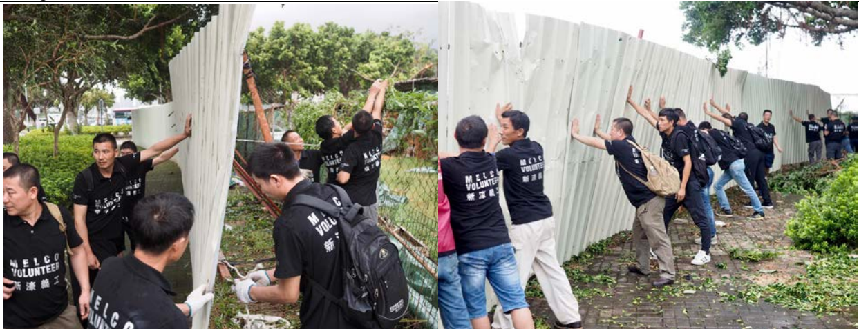
Photo 2 & 3: Melco team members fix broken hoarding in the city
